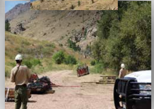
It takes a village...and a helicopter to haul in 600 pound beams and lumber for bridges. October, 2019
