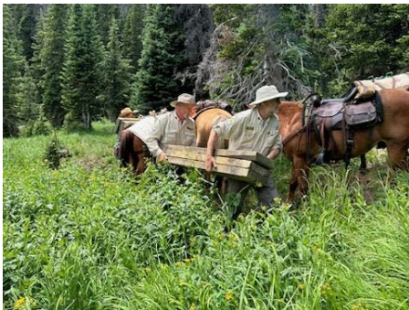
PWV members Tim Van Donselaar & Fred Allen unloading the deck planks at Rawah Bog
