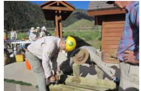
Preparations to begin carrying in the timbers needed to build a crib wall.
