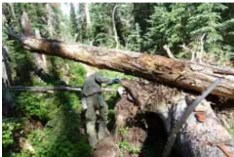
Downed trees present major obstacles for backpackers and stock on wilderness trails. PWV Trail Crew members spent five days in the Rawah Wilderness clearing trails.
